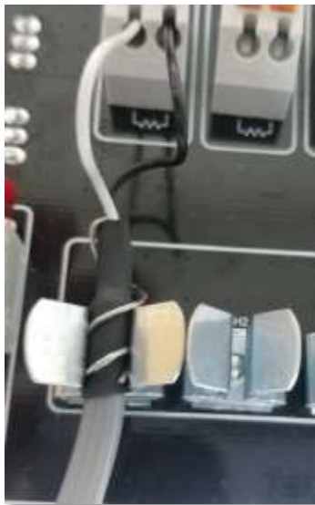
Figure 18: BOM cable inserted into 360° shield connection
