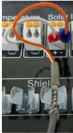
Figure 20: Solar irradiance sensor shield connection
